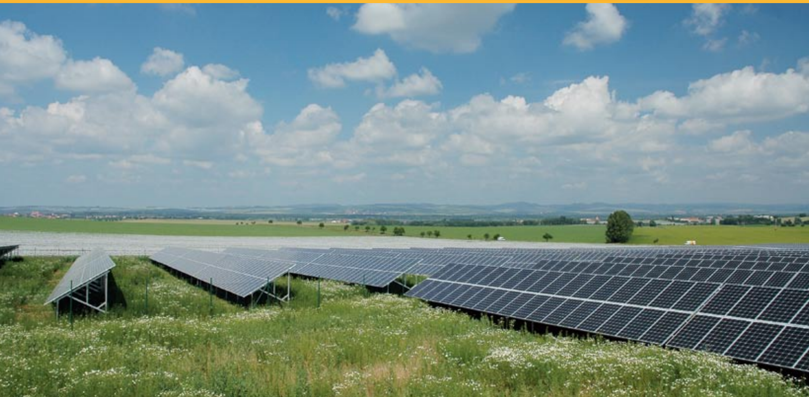
Solar arrays of Ostrožská Lhota power plant, Zlín region, Czech Republic; the power plant consisting of c-Si modules was constructed in the period 2007 to 2008 (courtesy: HiTechSolar)
