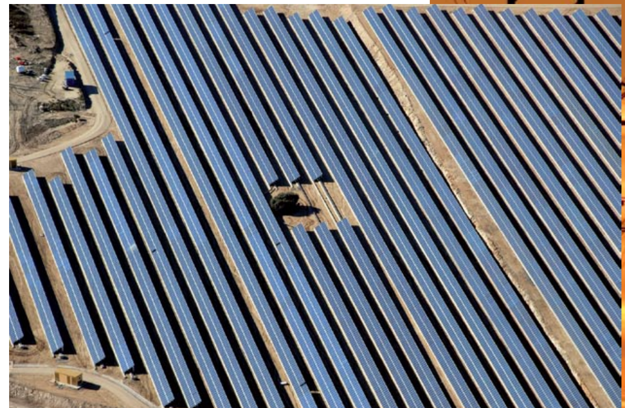
Solar arrays in Spain (courtesy: Suravia)
